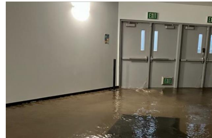
Figure 5: Flooded Hallway at CSU San Bernardino 4
