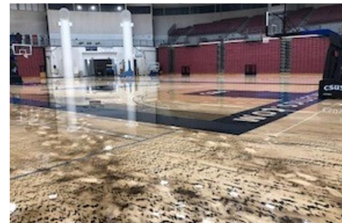
Figure 6: Flooded Gym at CSU San Bernardino
